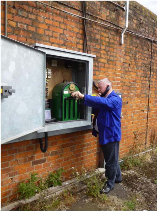
At Taunton a WSR driver speaks to the signaller at Exeter Panel and withdraws the token for the single line section to the West Somerset Railway, which also releases the junction signal allowing the train to run onto the heritage railway
